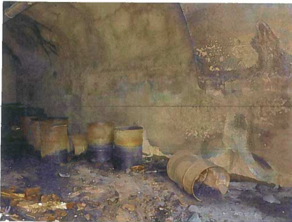
Figure 16. Interior of the magazine post-incident
